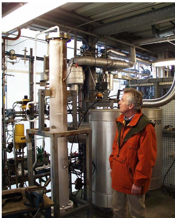
Fig. 2. Industrial scale desulphurisation filter for natural gas.
